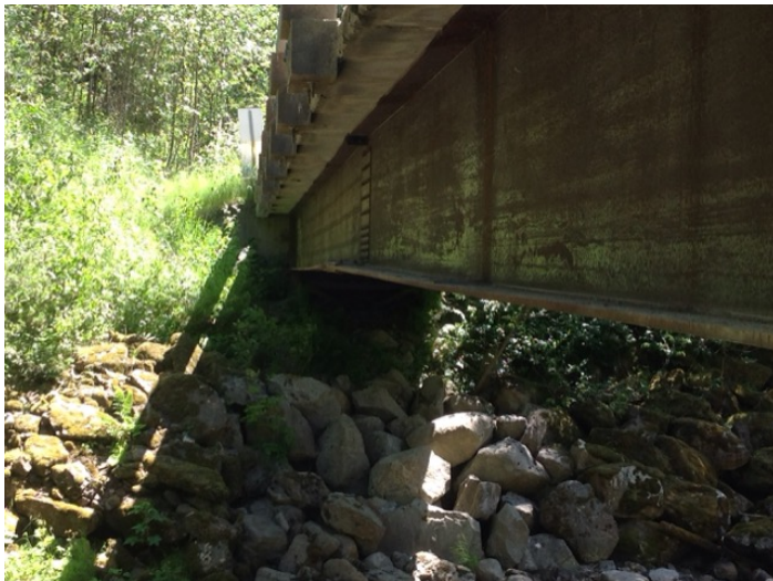
superstructure noticeably higher at splice
