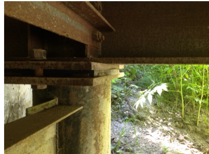
slight bulging on all bearing pads
